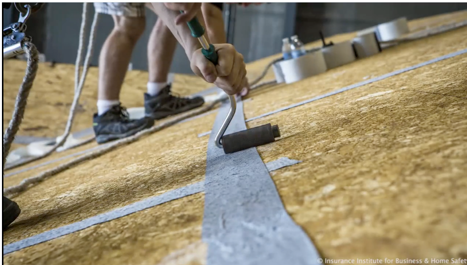
Figure 2-11. Installing a sealed roof deck system; taping the seams of roof sheathing.
